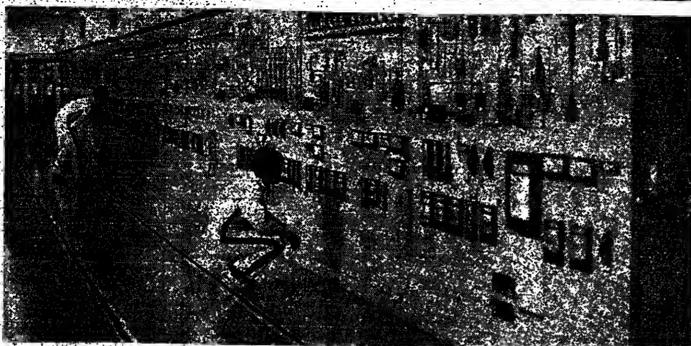
Computerised process controls are being increasingly used throughout industry. Above: the control room in the nuclear fuel reprocessing plant at Tokaimura, north-east of Tokyo. Safety is a key factor and surveillance must be constant
